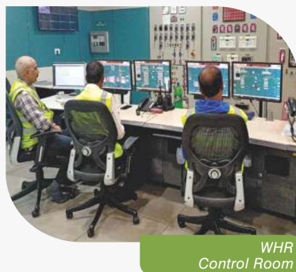
WHR at Narsingarh Plant
