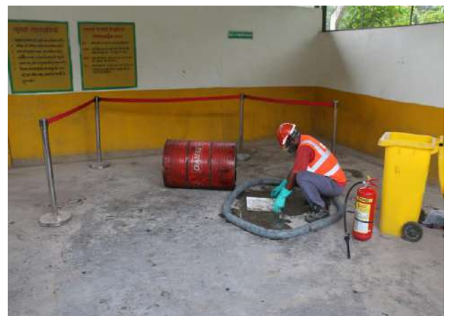
Used Oil and Grease spill trapping, having all necessary PPEs
