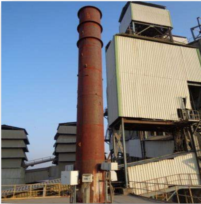
Photograph of CEMS Installed at Stack
