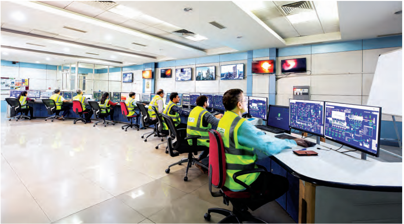
Plant operations monitored at the central control room at Narsingarh.
