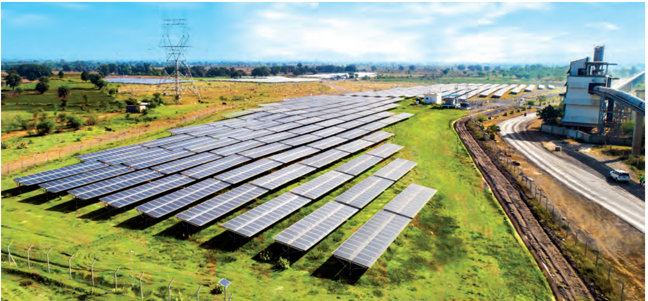
Recently commissioned 5.5 MW solar power plant at Patharia.
